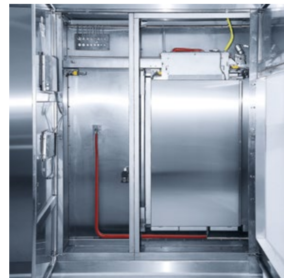
Airtight wall in stainless steel
