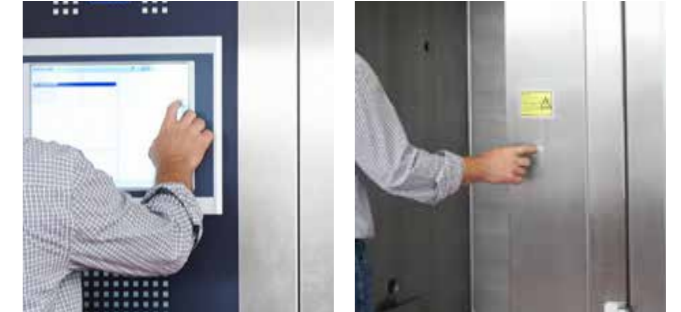
On walk-in chambers, additional safety buttons prevent people from being trapped.
