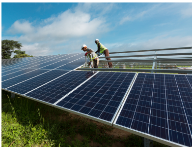
Senegal: Renewable Electricity from Solar Systems
